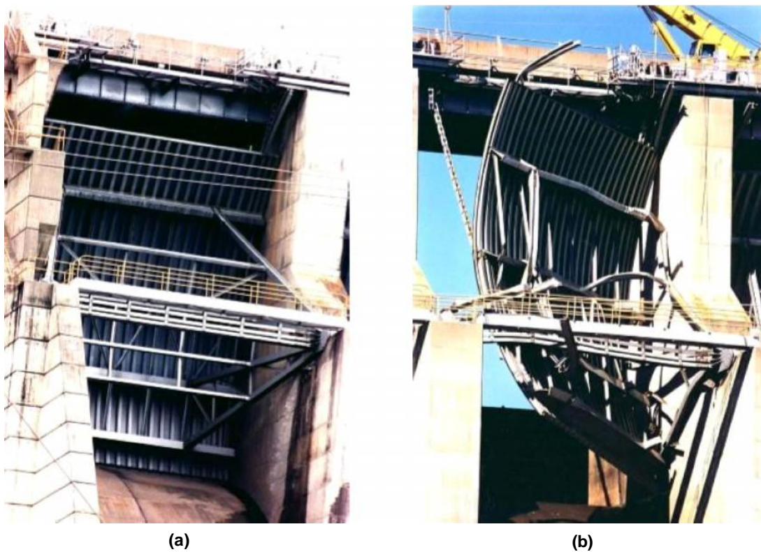
Figure 2: Two Views of Folsom Dam Tainter Gate: (a) Before Failure, and (b) After Failure
