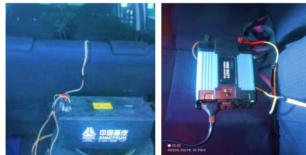
Fig. 9. 12V battery and AC to DC converter.
