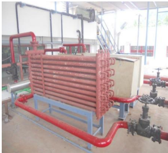
Figure 3: Refrigeration Heat Recovery Units
