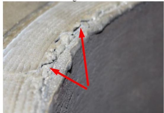
Figure 23. Cladding of cover plate (delamination of the coating)
