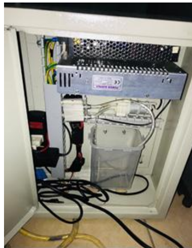
Figure 8. WCR prototype and control cabinet.
